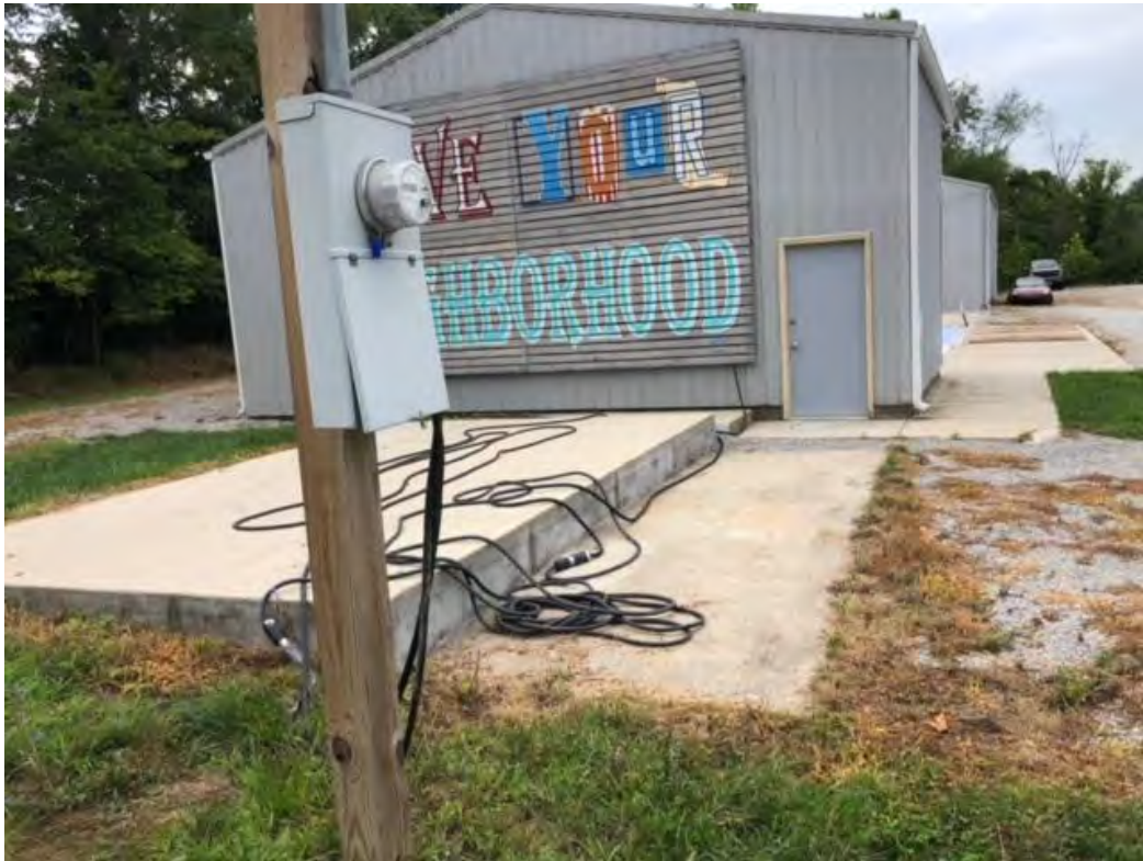
Photo 3. View of the building that was altered without permits August 2020. Photo by the Building Department.
